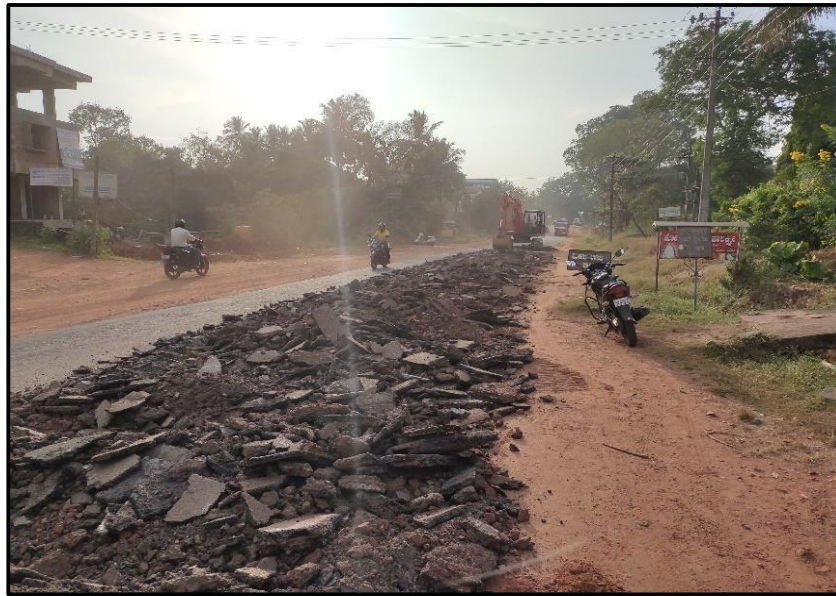
Fig. 3.4 Bulk RAP distressing from the NH169
