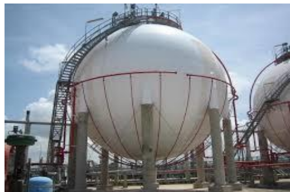
Fig 4: Unpressurized storage tank
