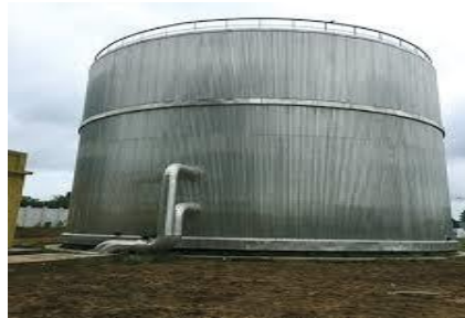
Fig 3: Unpressurized storage tank
