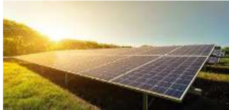
FIGURE 2: SOLAR PHOTOVOLTAIC (PV) ARRAY
