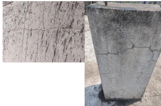
Fig. 3. Representative visual defects observed during inspection: (a) dampness/staining at a beam soffit; (b) hairline surface crack on a column face
